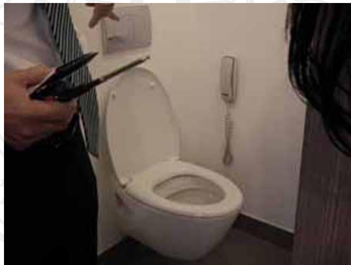
Figure 2.8 Toilet with dual flush system for water-saving use
